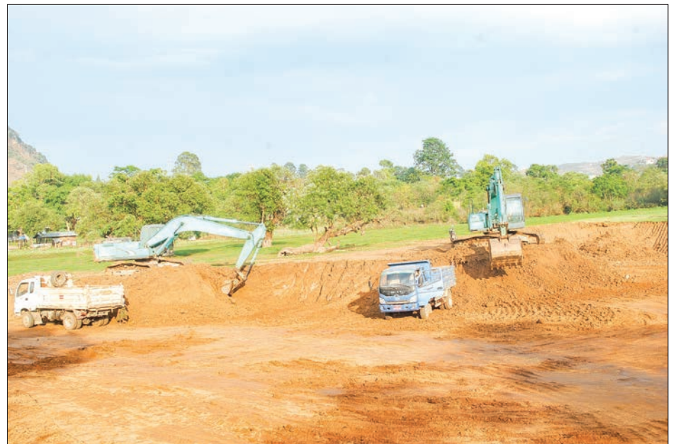
Machines digging the soil for Ganaing Pond (3) in Kyaung Gyi Su Quarter, Taunggyi, Shan State.
