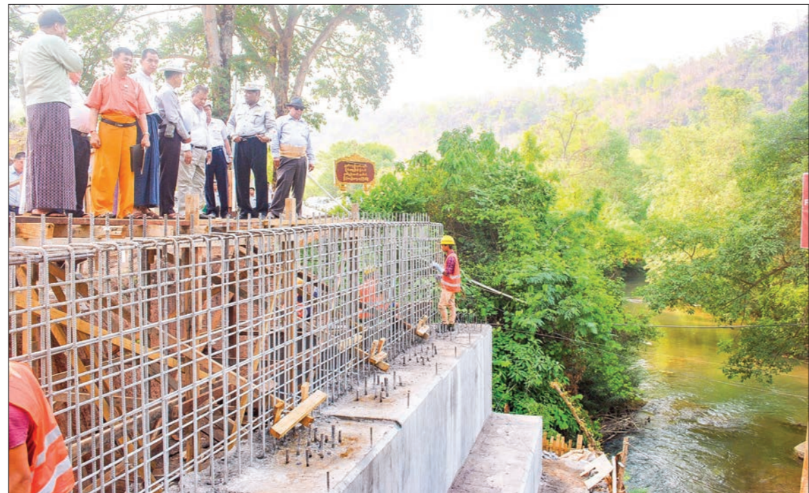
Shan State Chief Minister Dr Lin Htut and officials inspecting the construction of the Maukmai-Wunhat-Langkho Bridge.
