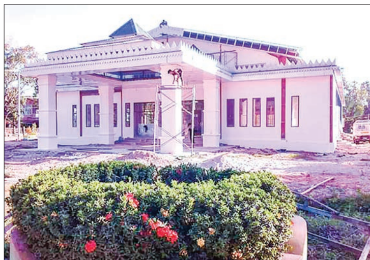
The City Hall being built in Indaw is nearly 100 per cent complete. PHOTO: LU AUNG (KATHA)
