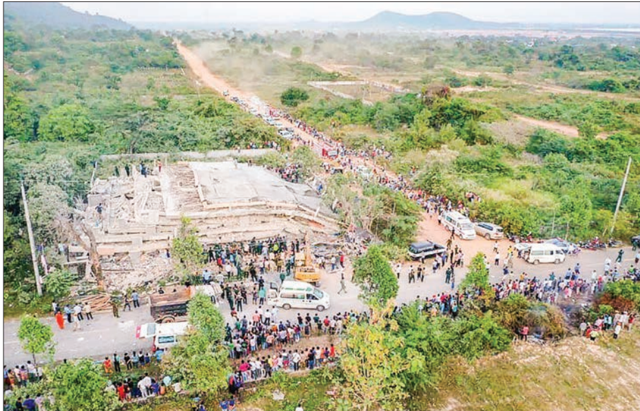
Supplied photo shows a building in the southern Cambodian town of Kep that collapsed and killed several construction workers. PHOTO: KYODO NEWS
