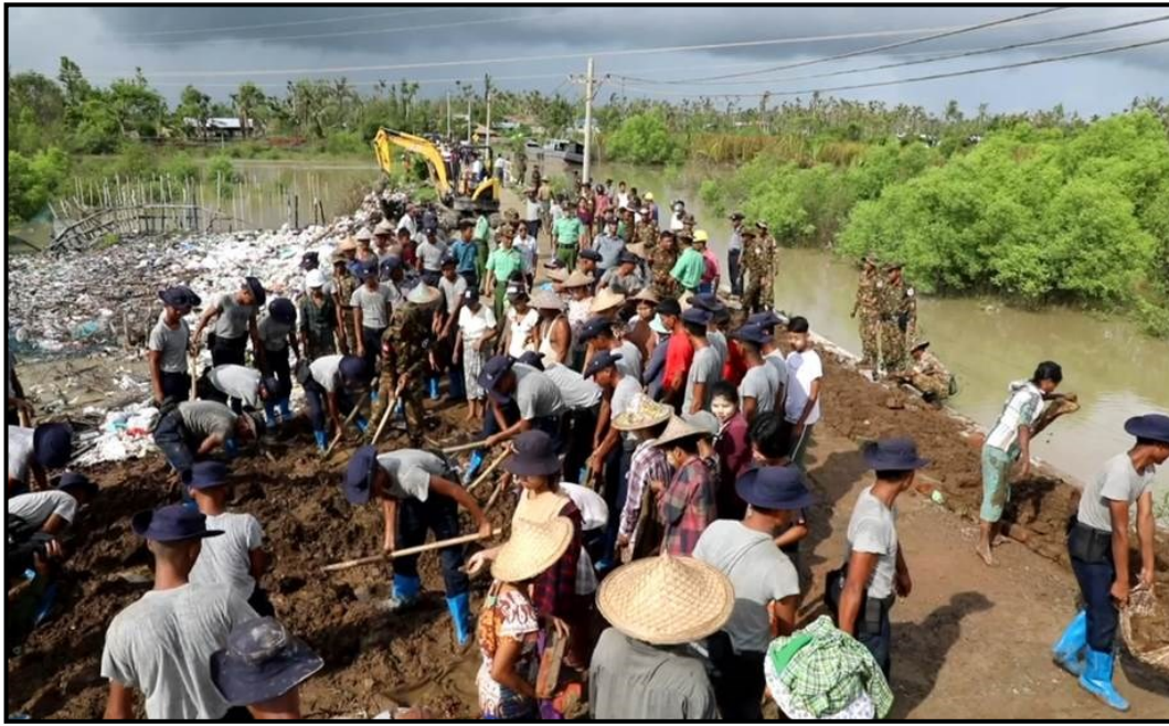
Collective activities of repairing the Ywathit Kay-Zaw Matak-Mingan Concrete Road in Sittwe by the relief and rescue teams together with locals
