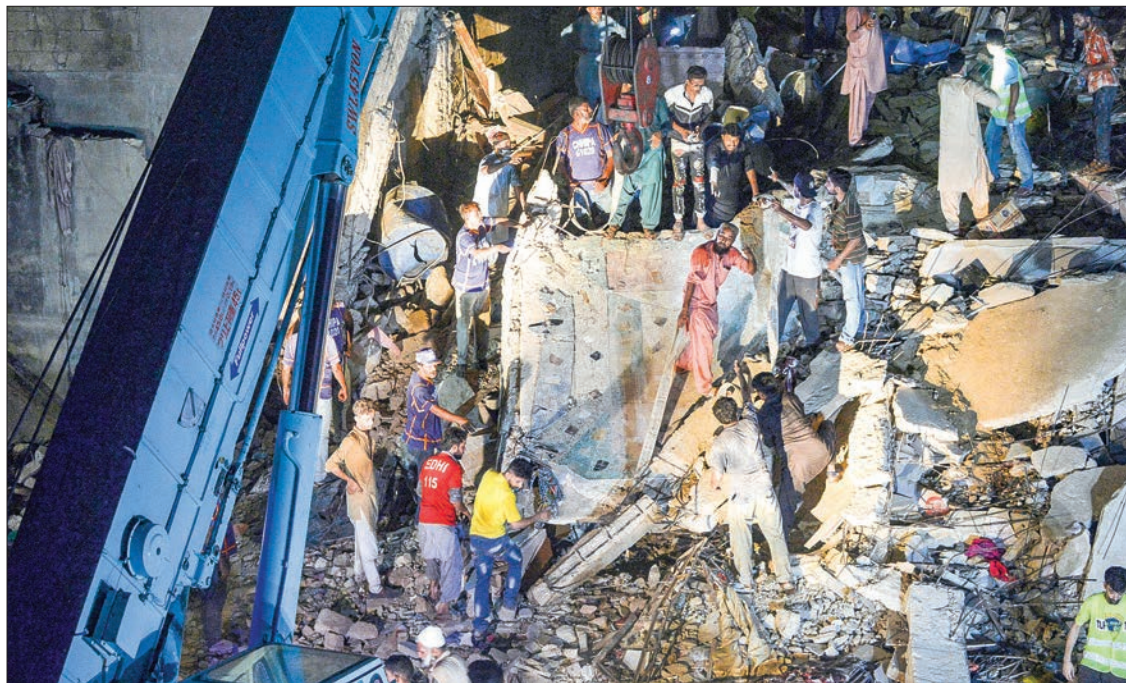
In this picture taken on 7 June 2020 rescue workers and residents search for victims in the rubble of a collapsed five-storey residential building in Karachi. PHOTO: AFP
