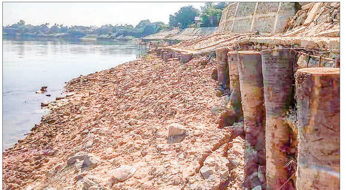
Over K5.3 billion worth riverbank protection project will be implemented next year.
